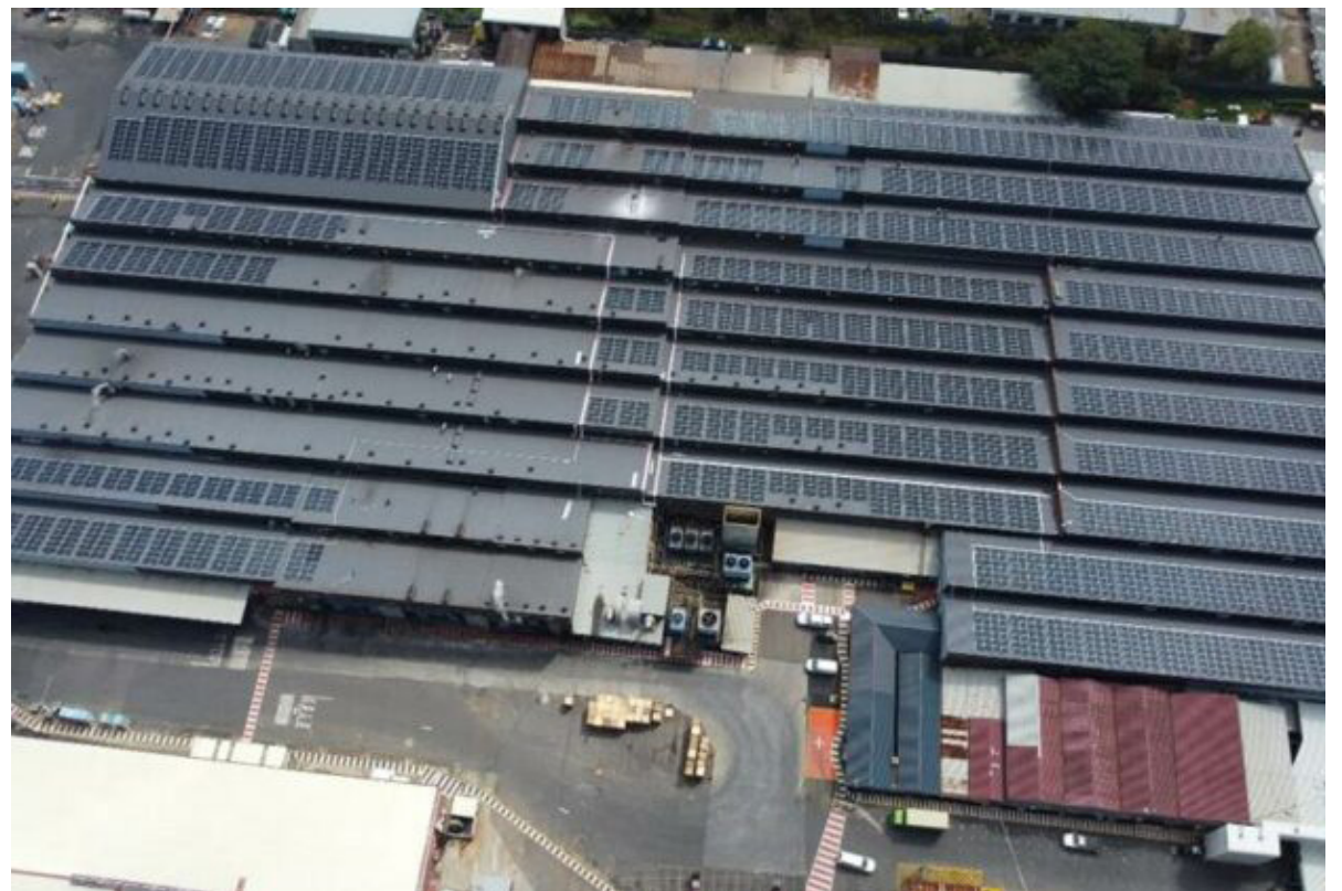
Solar panel installation at Tiger Brands’ culinary facility in Boksburg, Gauteng. -Photo: Supplied
