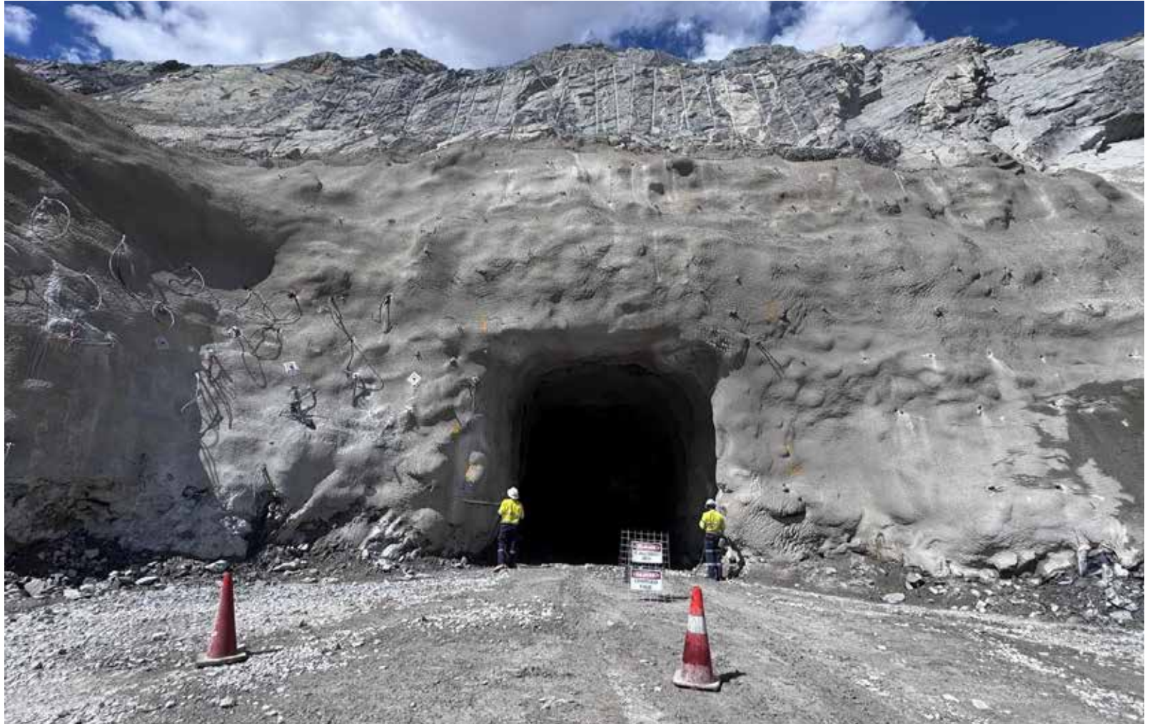
QKR Namibia Navachab Gold Mine is planning to start underground mining operations. - Photo: Contributed
